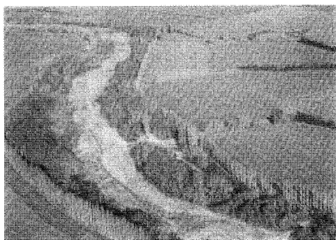
Figure 8.11 Bank protection by planted willows and poplars along the North Branch, Ashburton River.
