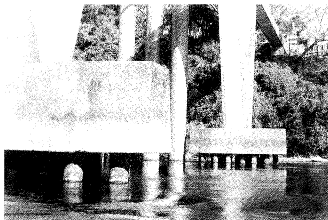
Figure 37.3 Piles exposed beneath the piers of the Claudelands Rail Bridge on the Waikato River, Hamilton.
