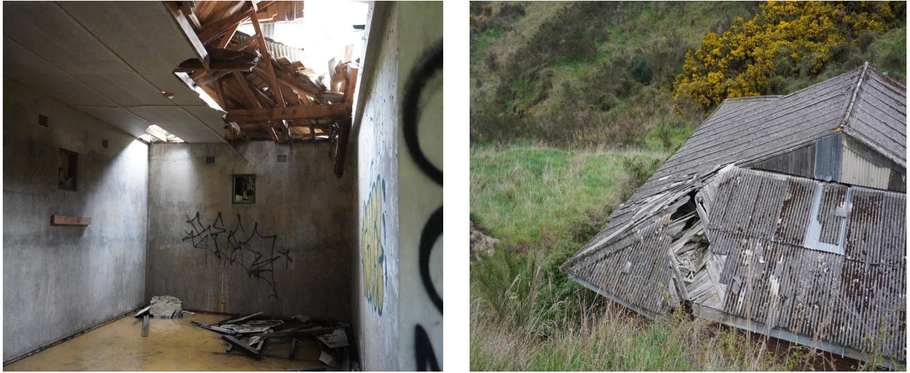
Figure 1. These images show the damage caused by rockfall to the bunkers in the Cass Bay Reserve.
